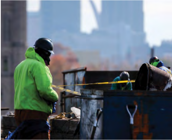
Lomax ensures that workers like these who are removing asbestos-containing materials from the Carter Carburetor site do so safely. Photo: Gene Watson, HRP.
